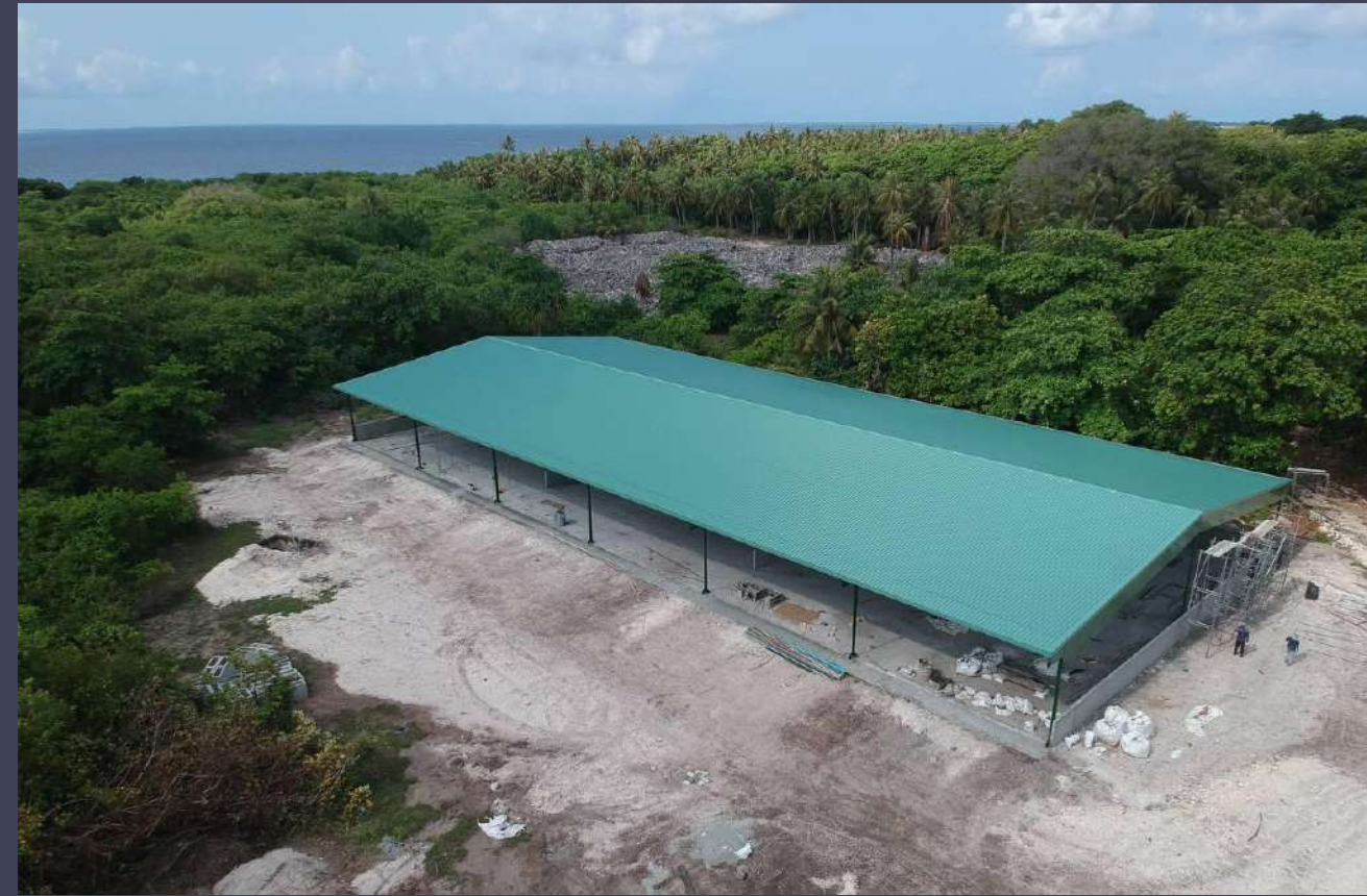
HDH. KUNBURUDHOO SOLID WASTE STORAGE SHED AND ACCESS RAMP COMPLETED DATE: 31-MAY-23
